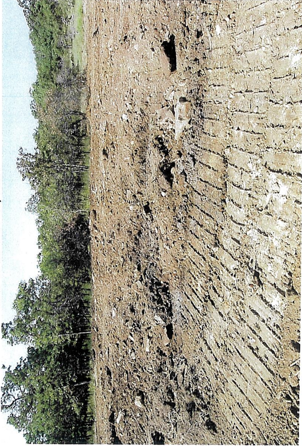
Photo 5 taken west. Close-up of soft and mushy area wet from pit soaked soils.
